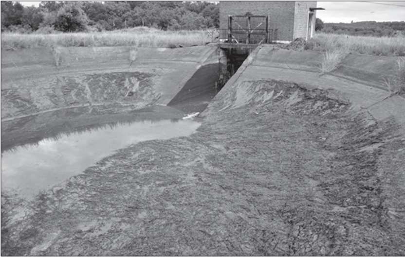
Damaged Siverskyi Donets — Donbas Canal. Photo: Korrespondent.net
